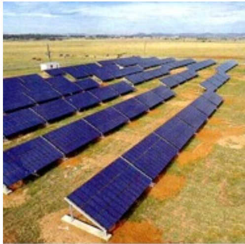
The Singleton photovoltaic solar array
